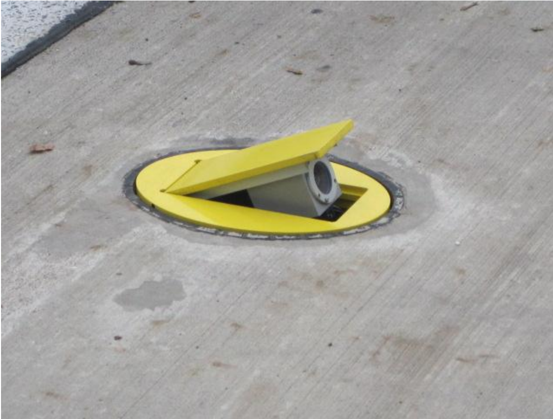
Figure 10 The next component in the system is an in-roadway thermal camera rig.
