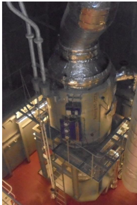
Figure 3. 13: Auxiliary EGE installed on board case ship
